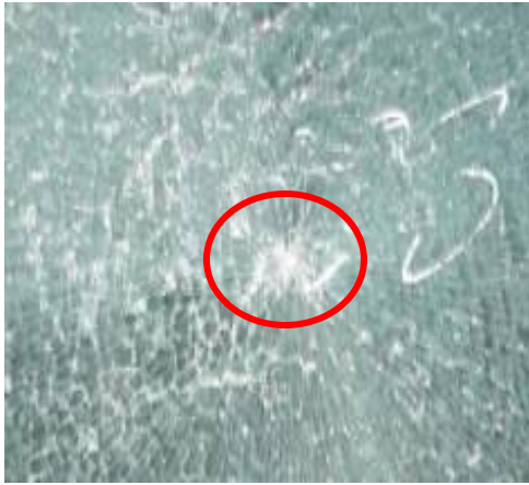
glass panel; glass is chipped at the crack initiating point.
