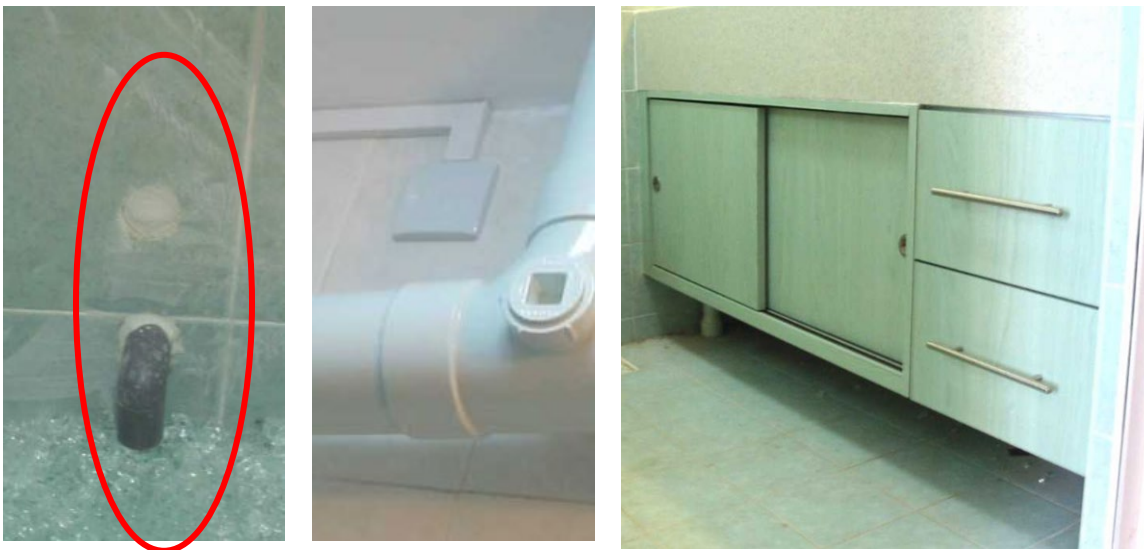
renovation work items; were carried out at the scene of the incident.
