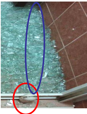
door hinges; the pivot is in 'close' position but the door panel debris indicates it was open during the incident.
