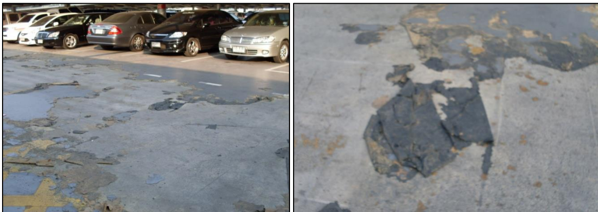
Figure 2 Delamination of Waterproofing Membrane in Thailand Airport Carpark (Fosroc)
