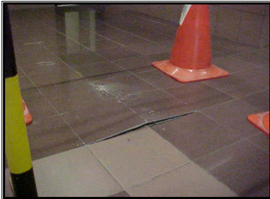
Photo 1 - Arching and lifting of floor tiles
