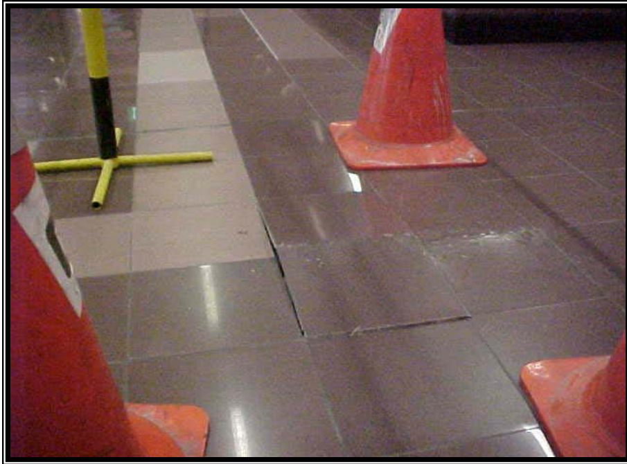
Photo 2 - Another view of the defect
