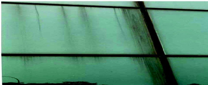
Figure 3.43. Staining on glass originating from open joints.
