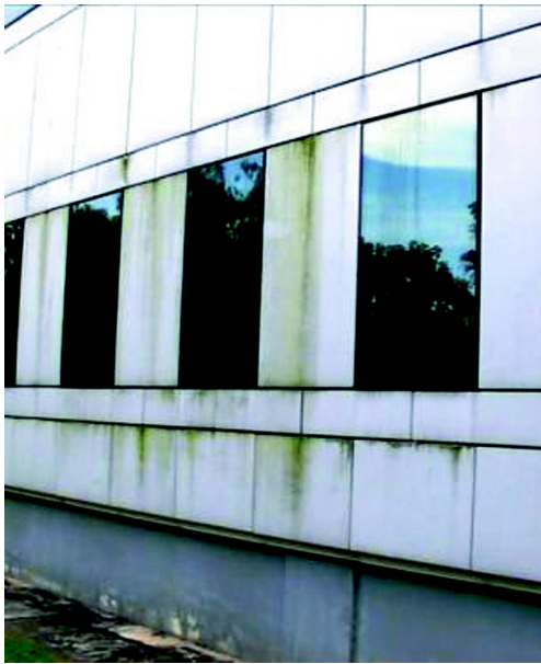
Figure 3.38. Biological growth on facade at ground level and in proximity to vegetation.
