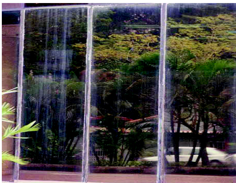
Figure 3.47. Staining of glass due to corrosion of sealant.
