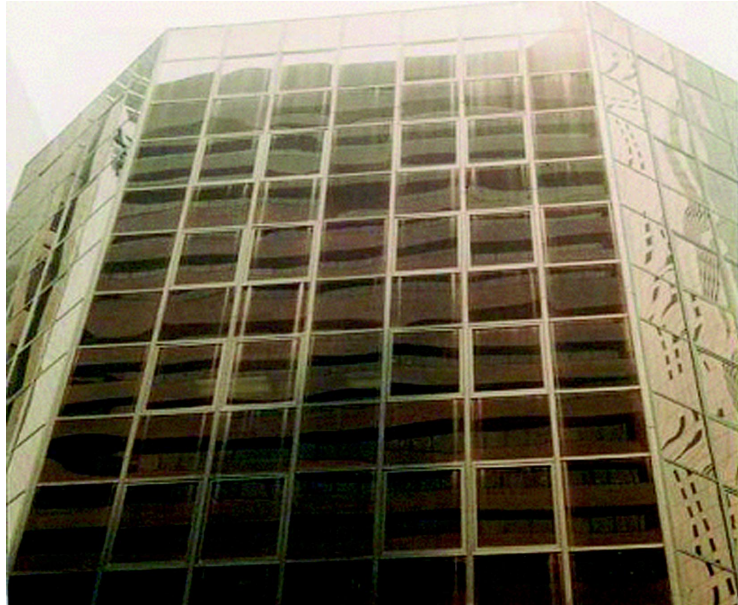
Figure 3.49. Staining from weepholes results in a regular staining pattern throughout the facade.
