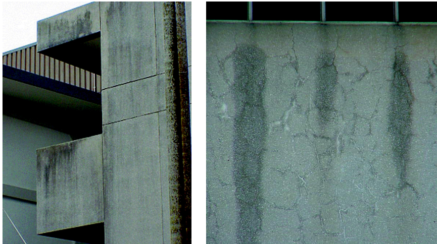
Figure 3.51. Dirt staining of Shanghai plaster.
