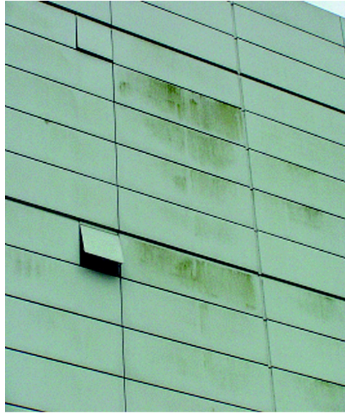
Figure 3.39. Biological growth on facade panels at 4th storey and in proximity to trees.
