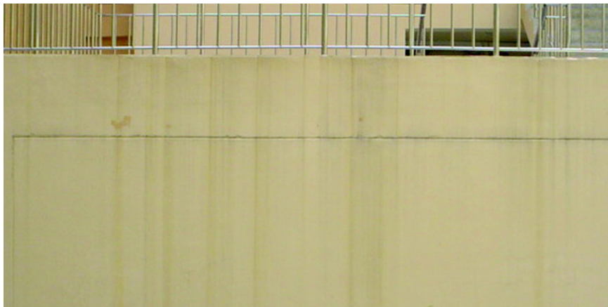
Figure 3.52. Dirt staining on a smooth plaster-and-paint wall.
