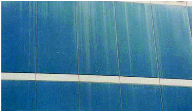
Figure 3.36. Staining on enamel steel resulting in corrosion of panels.
