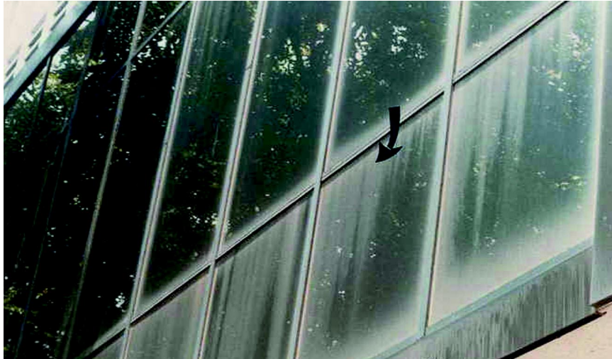
Figure 3.48. Staining of glass due to corrosion of transoms and mullions
