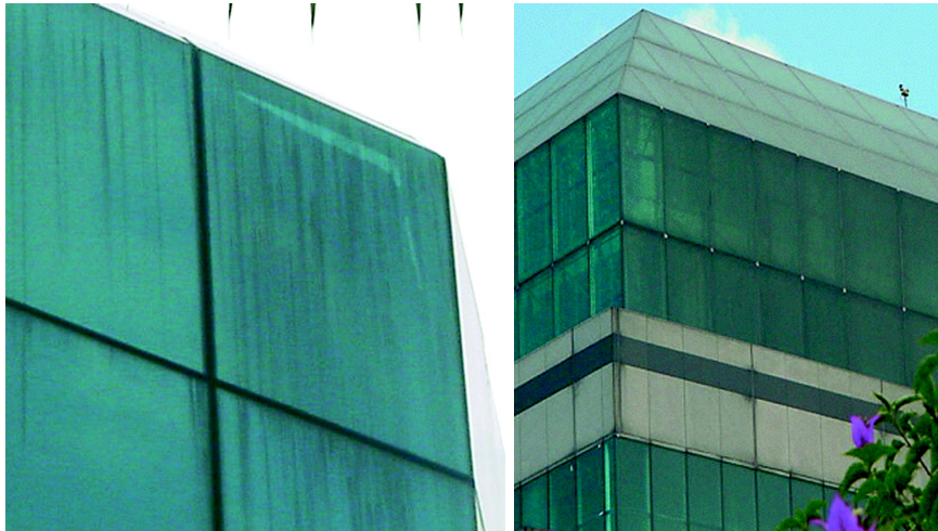
Figure 3.44. Accumulation and washing off of dirt from the sloping roof causes staining on the glass facade.
