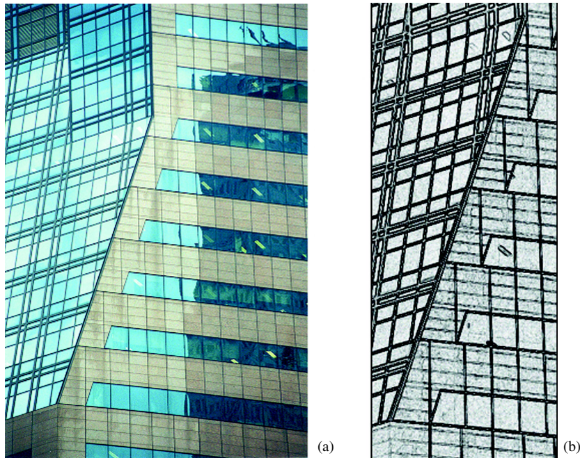
Figure 4.26. (a) Joints misalignment on the facade of the building interrupts the even flow of runoff and results in staining. (b) Drawing shows the clear misalignment of joints.
