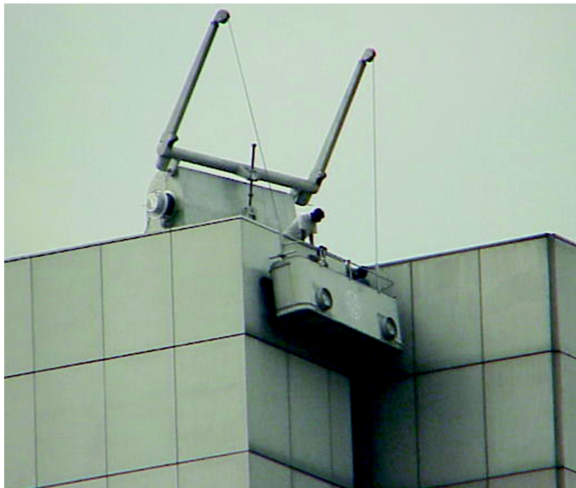
Figure 5.8. A trolley unit suspended from a lifting hoist running on the roof.
