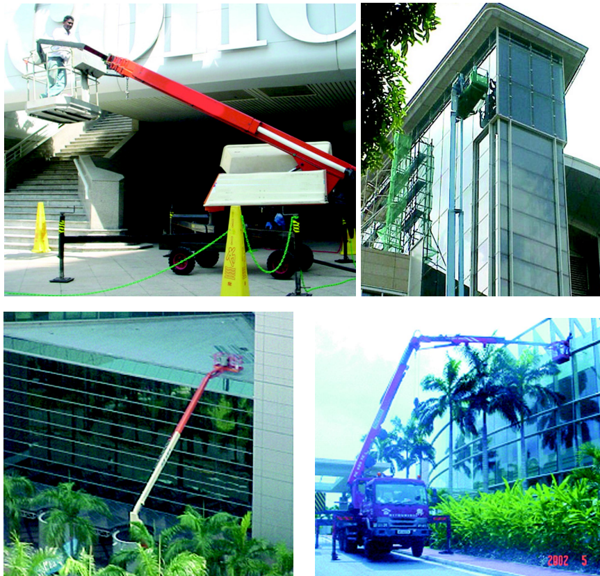
Figure 5.24. Articulated boomlifts for external facade's maintenance.
