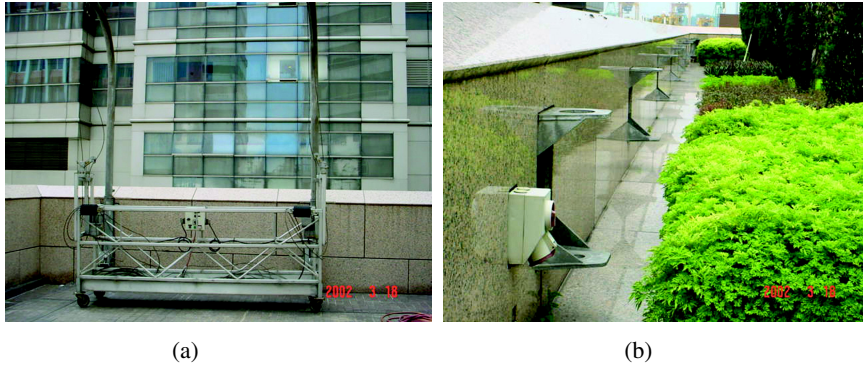
Figure 5.15. Platform suspended from fixed davits.
