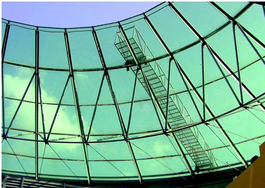
Figure 5.17. Traversing ladder with fixed guardrails for cleaning the exterior of a glazed roof.
