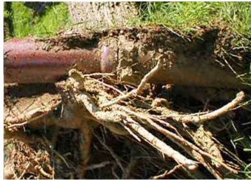
Figure 2&3: Root Damage to Drainage and Pipe
