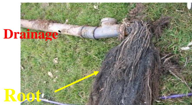
Figure 4: Pipe blockage caused by plant roots
