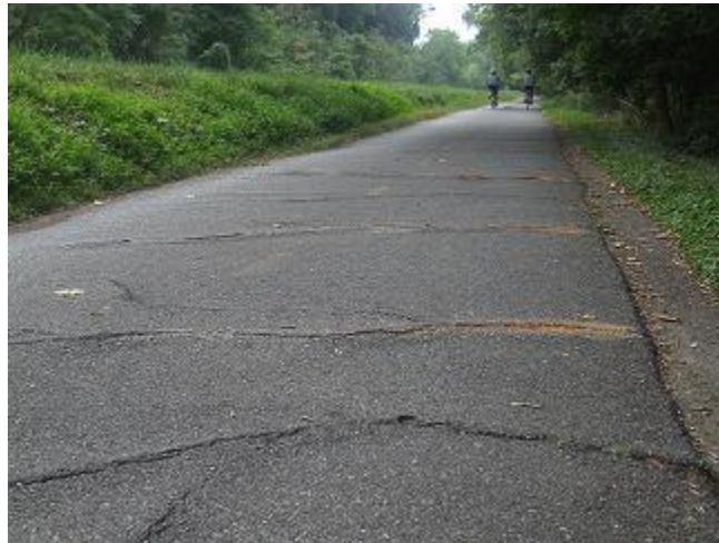
Figure 1: Root Damages to Pavement
