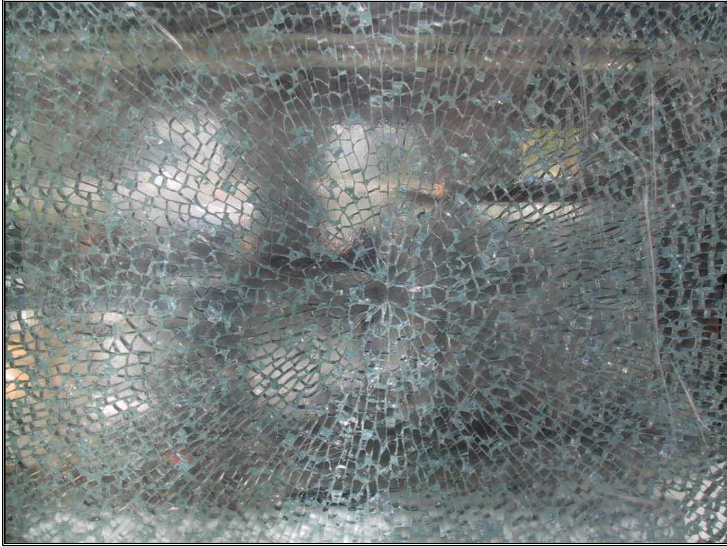
Figure 1: Sun-burst crack pattern of spontaneous breakage caused by expansion of Nickel Sulphide inclusion
