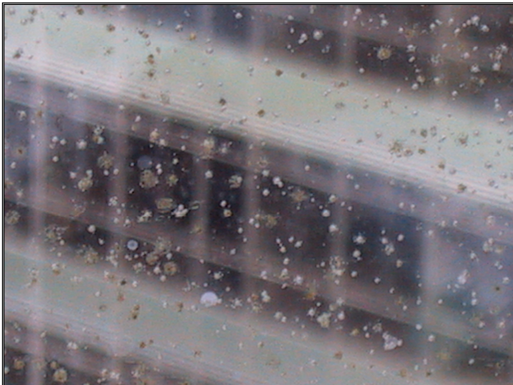
Figure 6: Typical weld splatter on glass
