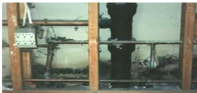
Figure 21: Plumbing Vent Stack
