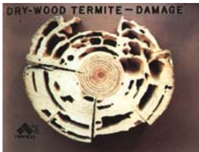
Figure 24: Typical drywood termite damage. Note that the galleries are extensive and that they cut across several annual rings.
