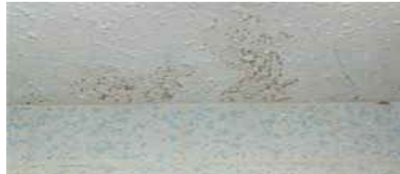
Figure 18: Subterranean Termites In Ceiling
