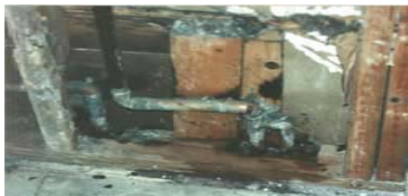
Figure 19: Plumbing Line In Wall
