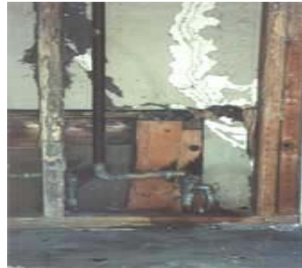
Figure 20: Plumbing Line In Wall
