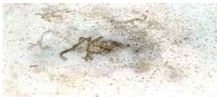
Figure 17: Subterranean Termites In Ceiling
