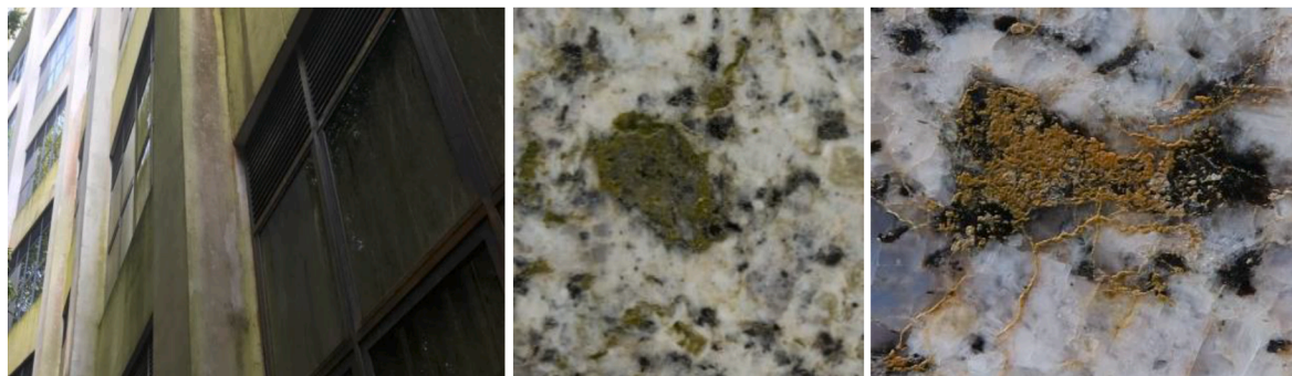
Fig. 1. Biological growth on external façade.
